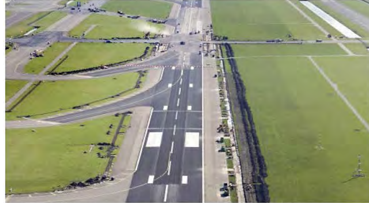
Overview of the paving project at the Polderbaan, with Cargill's Anova® Rejuvenator. © 2021 Heijmans
